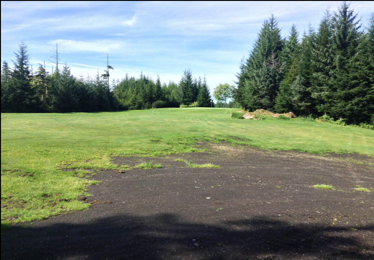
Construction continues on fairway #3. USGA allows for a free drop out of the "ground under construction" area.
