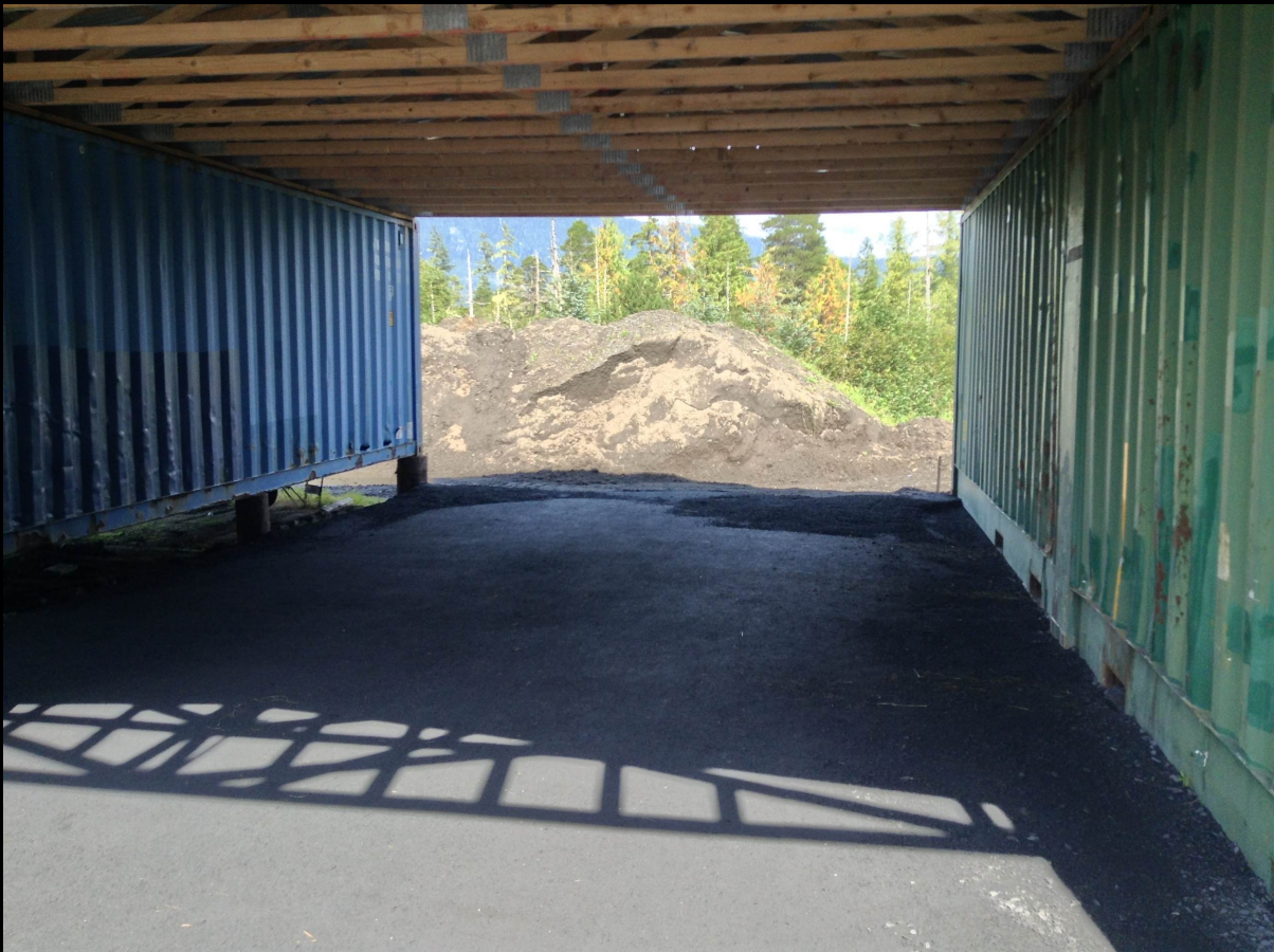
Phase two of the covered motor cart garage has begun. Pictured above is the inside after flooring was installed. Custom built doors by Lloyd Ward will be installed on either side of the garage for easy access to personal motor carts.
